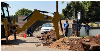
GENERAL BUILDING | 5GB
